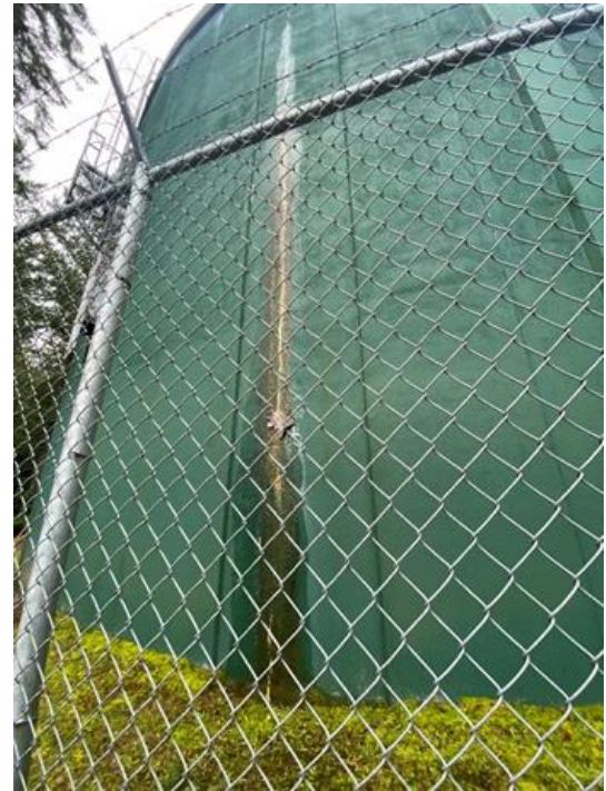
Figure 5: Large municipal tank indicating leak and surface corrosion. (Credit: N. Elmieh)
