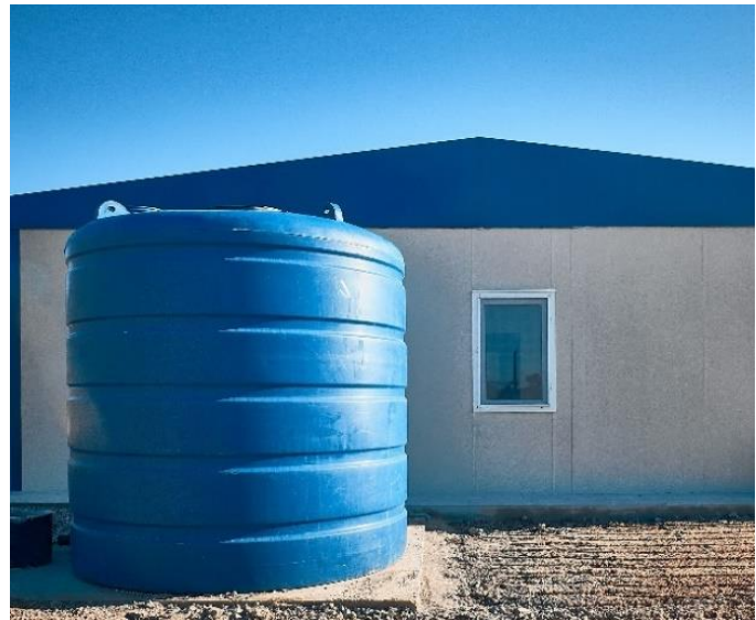
Figure 2: Water storage tank on concrete plinth supplying a temporary site.
